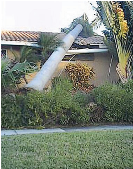
Figure 10. Roystonea regia (royal palm) fallen on house because the trunk was weakened from Ganoderma butt rot Credits: Ted Conner Landscaping
