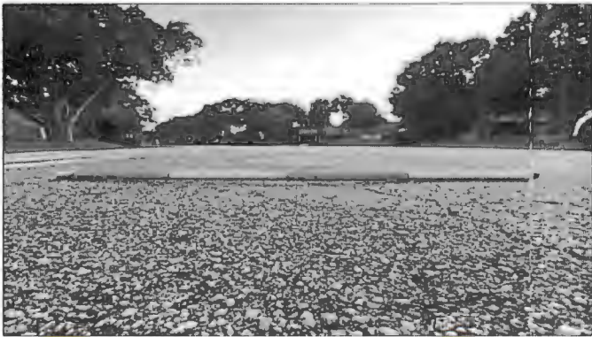
Hammocks Blvd – Rutting
