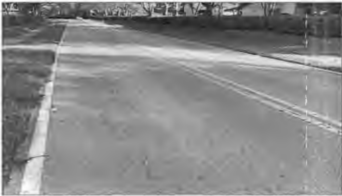
Carambola Cir N – Linear Cracking
