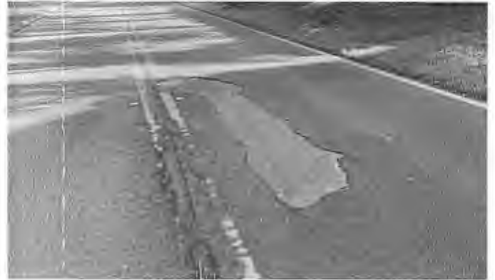
NW 42 nd Ave – Raveling
