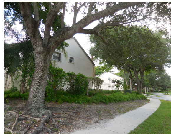
Bare areas and grading issues along NW 22nd Road.
