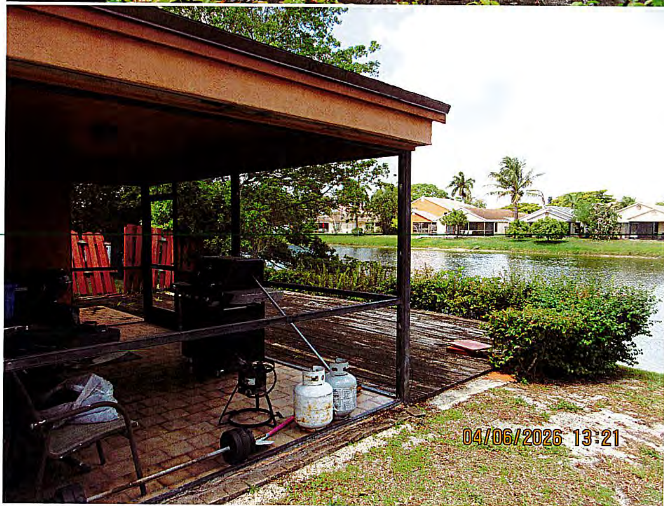
3411 NW 21 St (Centura Parc) Observed fence & deck in disrepair. 4/6/26: 1:21PM JM
