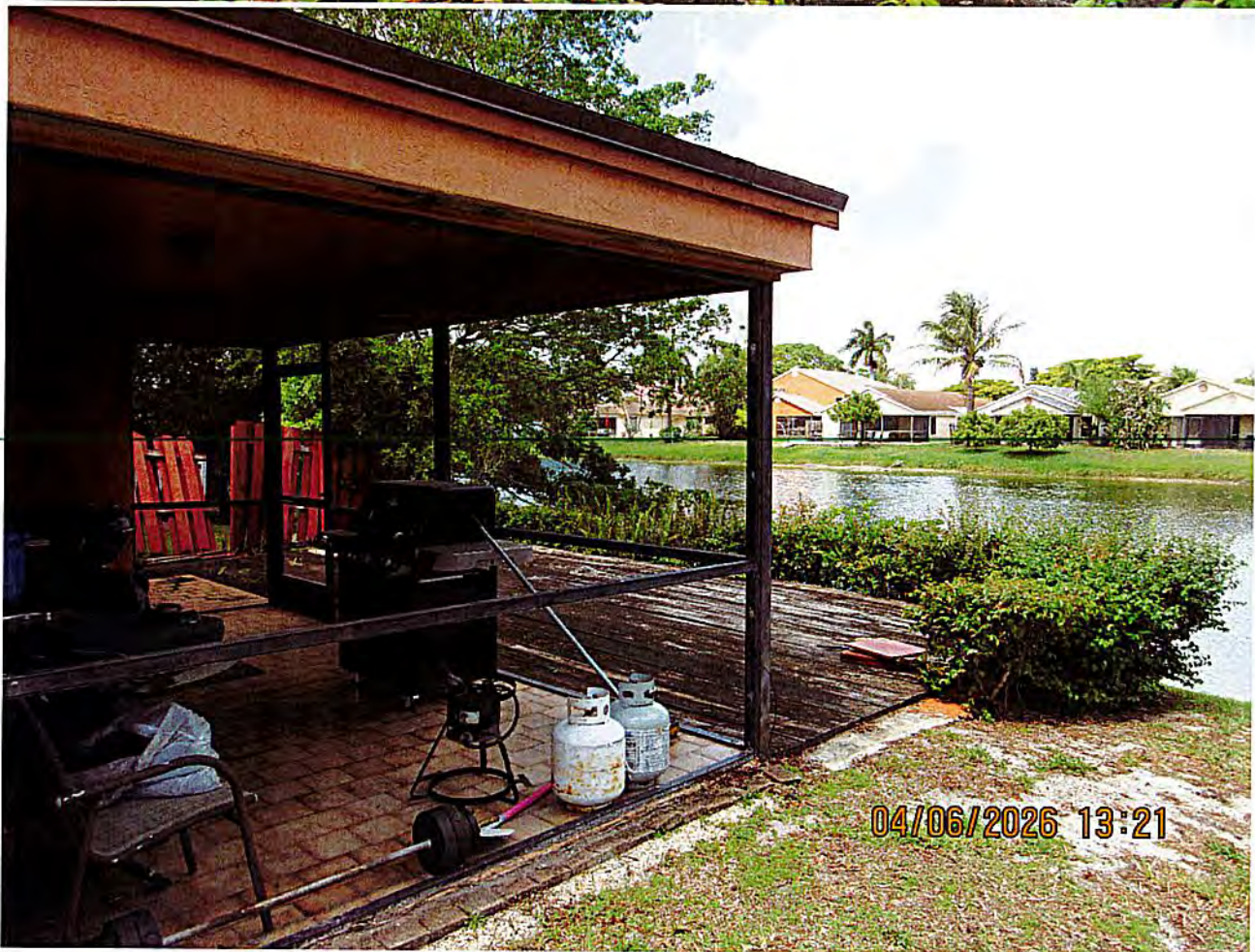
3411 NW 21 St (Centura Parc) Observed fence & deck in disrepair. 4/6/26: 1:21PM JM
