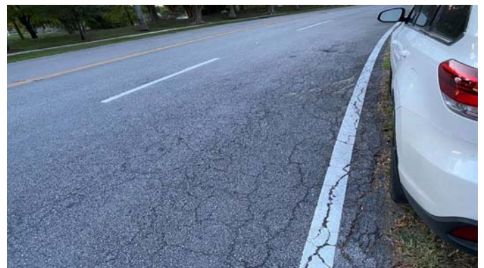
Hammocks Blvd – Alligator Cracking and Edge Cracking
