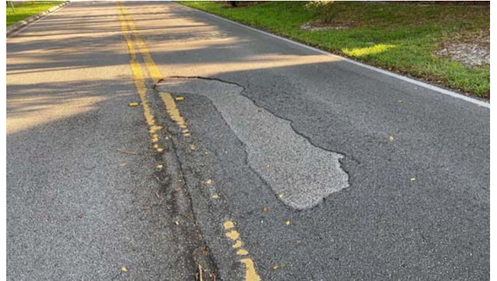
NW 42 nd Ave – Raveling
