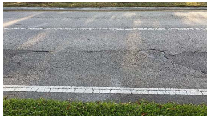
NW 42 nd Ave – Raveling, Alligator Cracking and Patching
