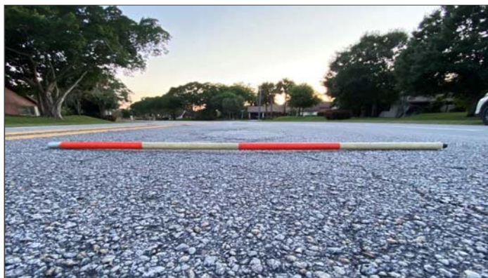
Hammocks Blvd – Rutting
