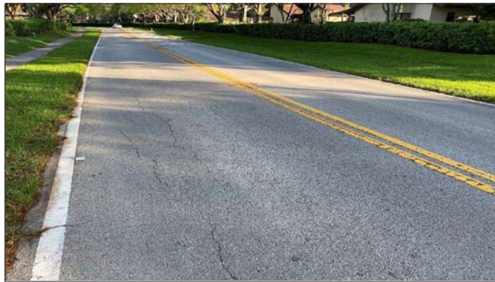
Carambola Cir N – Linear Cracking
