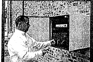
Rack Enclosure mounted on a wall
