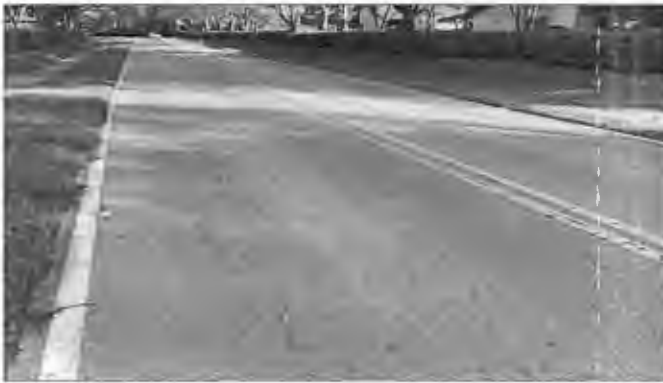
Carambola Cir N – Linear Cracking
