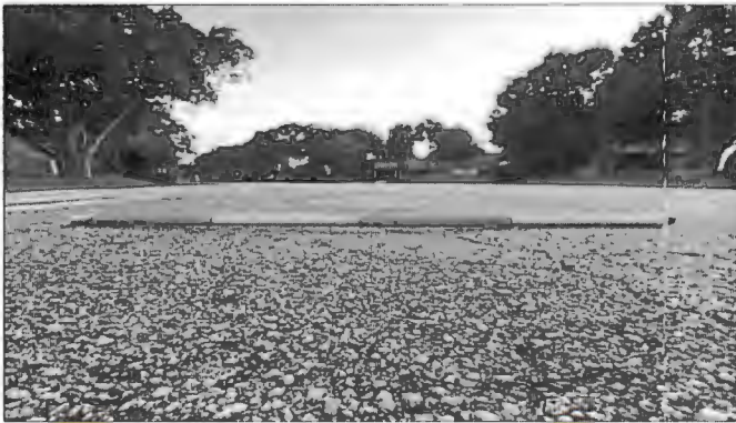
Hammocks Blvd – Rutting
