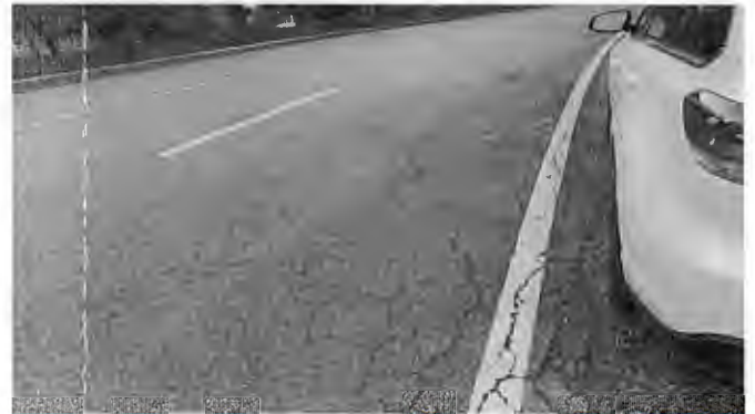
Hammocks Blvd – Alligator Cracking and Edge Cracking
