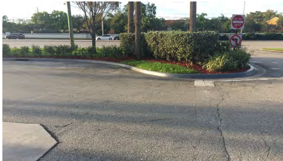
Pavement marking faded at the right-in only entrance (Looking South)
